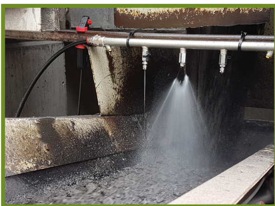
Figure 4 – Addition of rejuvenator to RA on the conveyor belt by means of a spraying system (source: BRRC [21])
