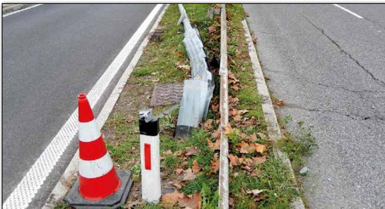
Figure 1 – Poteau de sécurité passive percuté (source: Safety-Product)
